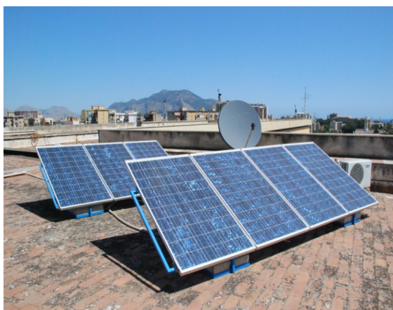
Fig. 3 – 2x3 PV plant (one module disconnected)
